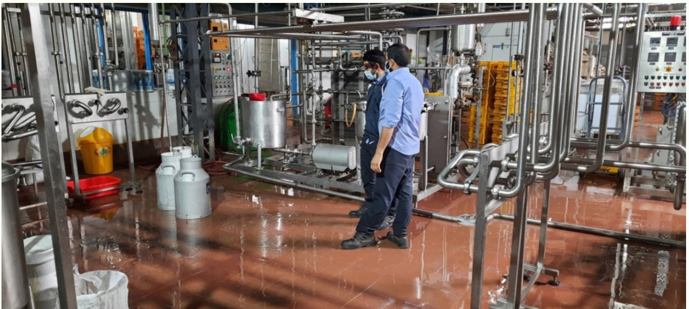
50 Thousand Litres per day Milk Processing Plant at Cheshmashahi, Srinagar-NPDD scheme
