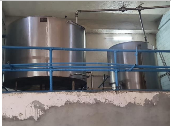
Ghee Storage Tanks
