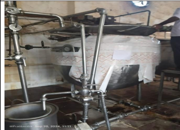
Ghee Settling Tank
