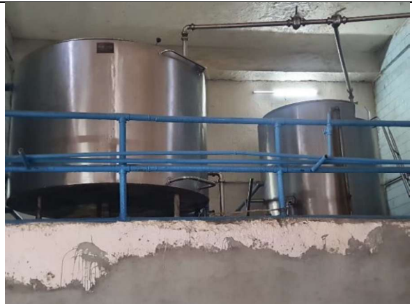
Ghee Storage Tanks
