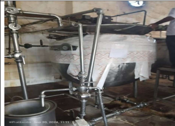
Ghee Settling Tank
